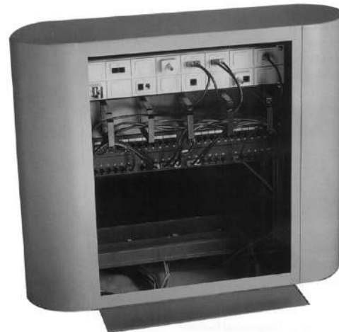
Fig. 13. Distributed satellite closet serving 10,000 sq. ft. (930 sp. meters) offer greater control, reliability and flexibility to meet individual needs (POWERFLOR™).
