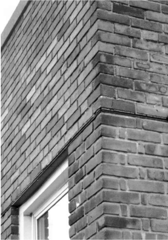
Fig. 5. Brick masonry cracked by expansion of carroding
