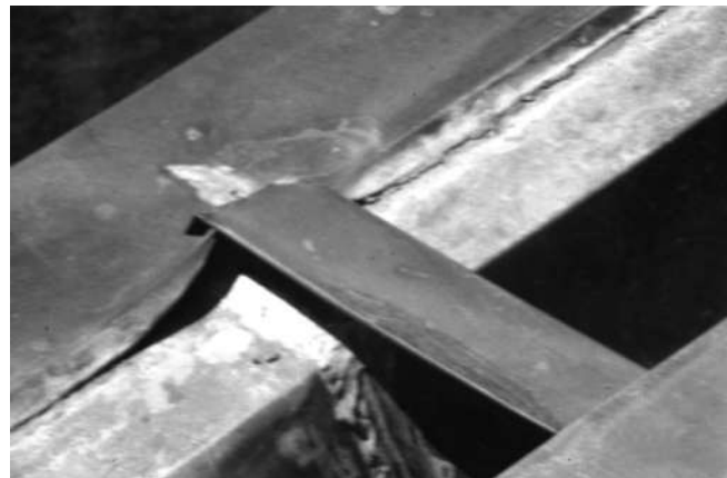
Fig. 15. Expansion joint not properly constructed; moving elements join fixed elements rigidly, and the joint has twisted and broken.
