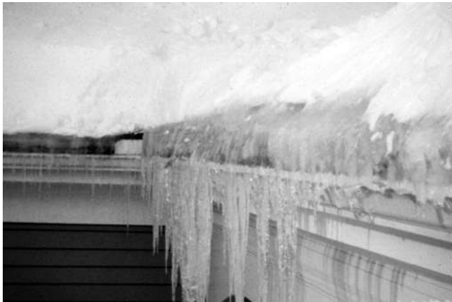
Fig. 14. Ice dam at eaves of steep roof. Thick deposit of ice causes melt water to back up and run through laps and joints in shingle roof. Eave flashing is intended to tolerate ice damming and prevent melting water from entering building.
