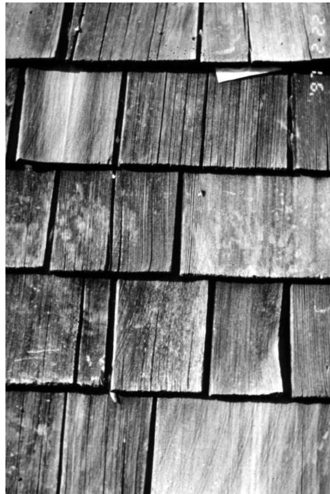
Fig. 12. Split shingles: the first and third course joints lined up in many places. When the intermediate shingles split, there was a clear path through the shingles for rain water.)
