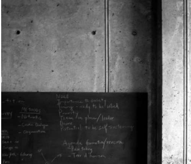
Fig. 10. Interior detailing of concrete form joints. Salk Institute, La Jolla, CA. Office of Jonas Salk. Louis Kahn, Architect.
