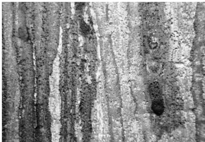
Fig. 6. Pitting and corrosion of copper flashing as a result of runoff from membrane roof.
