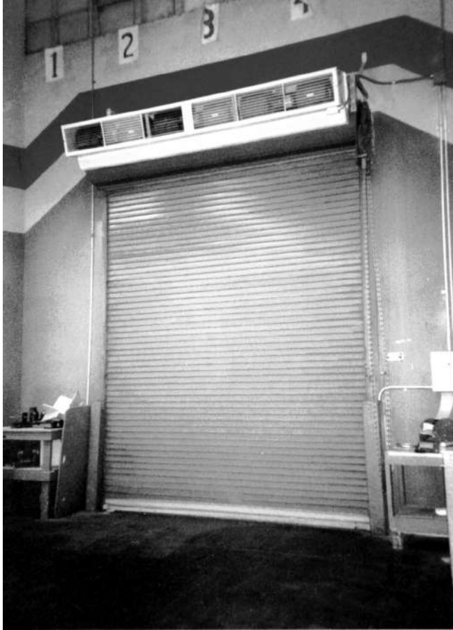
Fig. 4. Air curtain installed over bay door on interior of loading dock. (Courtesy: Mars Air Door)
