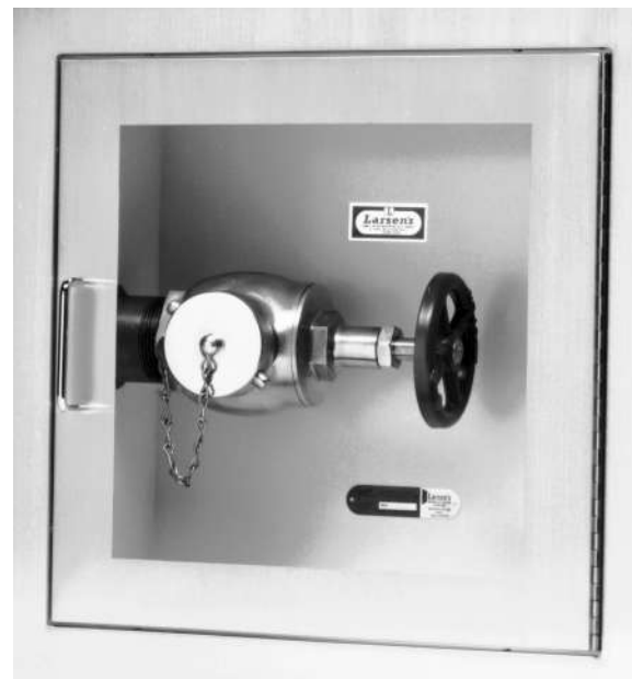
Fig. 1. Standpipe valve in recessed cabinet
