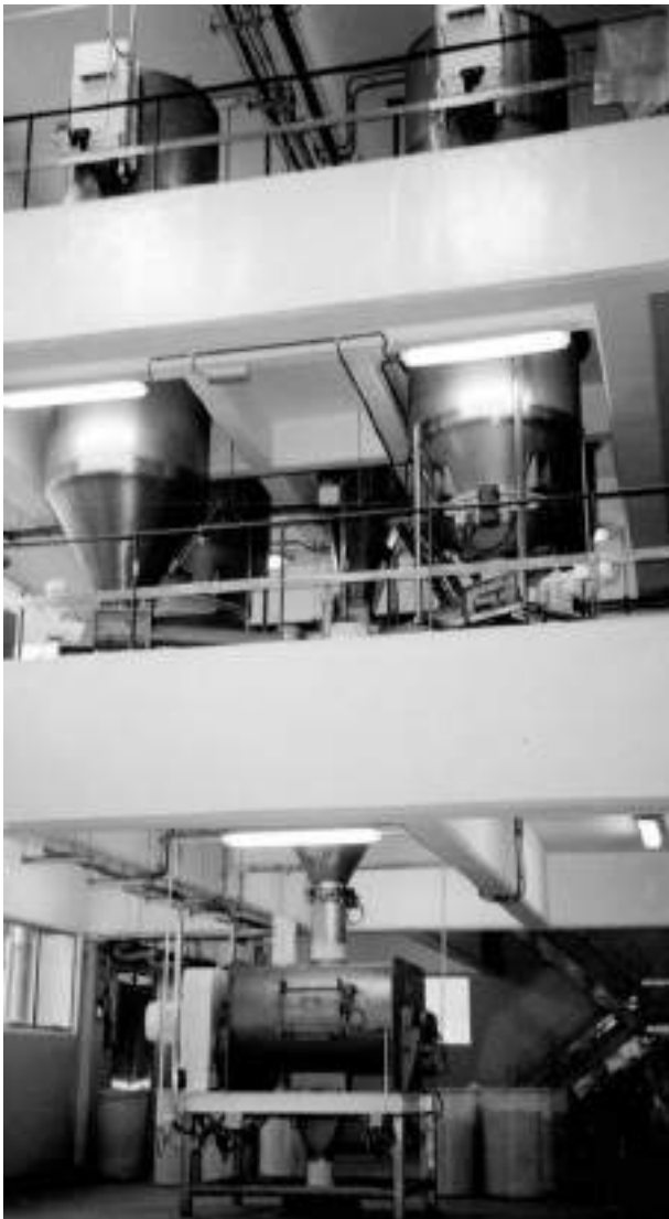
FIG. 21-52 Classical automated batch mixing installation. The components are stored in small silos shown at the top of picture. The materials are extracted from these hoppers in a downstream weighing hopper according to the recipe. Once all components are fed into this weighing hopper, a valve is opened and the exact batch falls into the downstream batch mixer.
