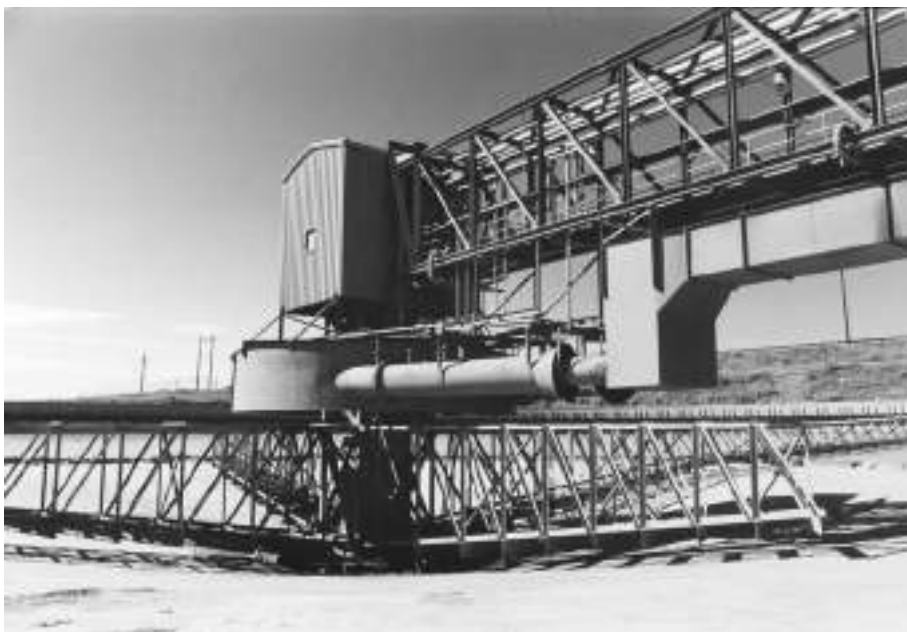
FIG. 18-105 E-Duc® Feed dilution system installed on a 122-m diameter thickener. (Dorr-Oliver EIMCO.)
